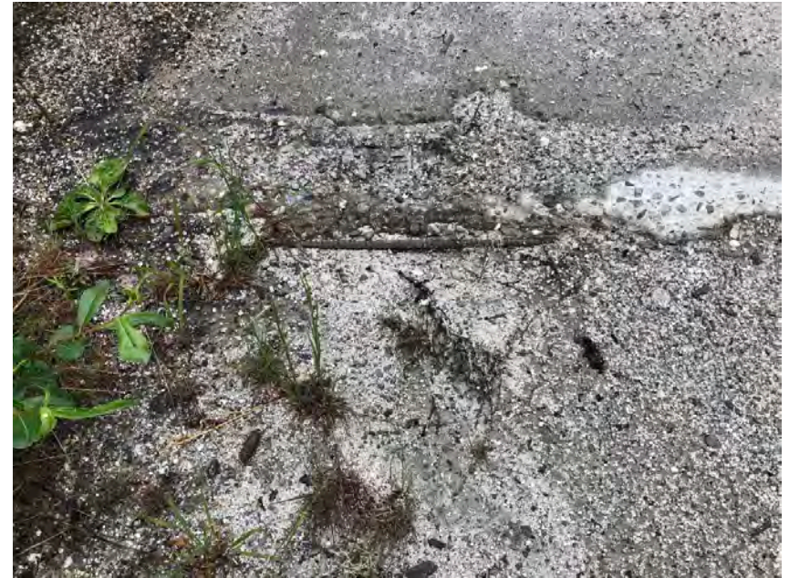
Damage noted to ballast wall at road surface
