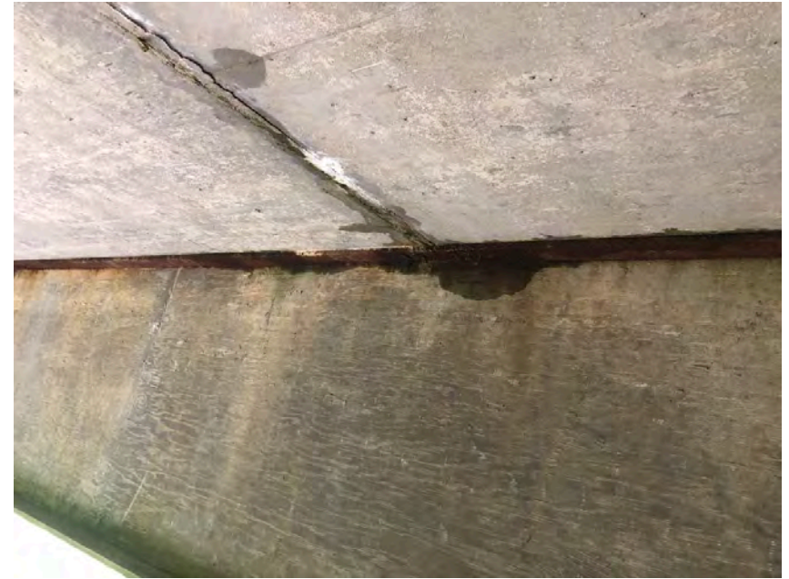
Evidence that water is getting through some deck joints
